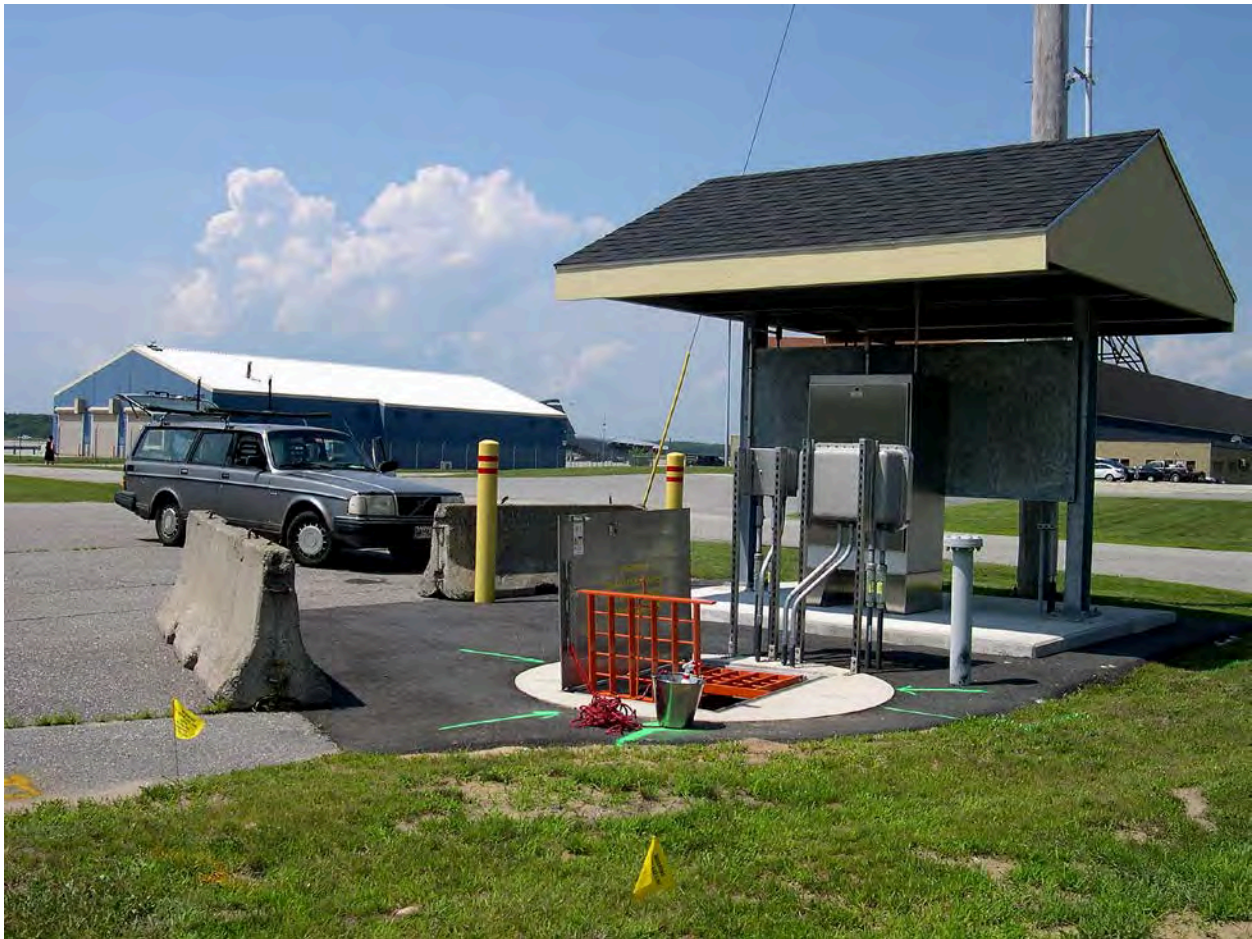
Public Works Pump Station
